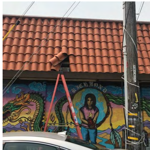
Roof tiles moved to reveal rodent access behind
