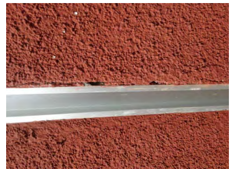
Small gaps in stucco that had to be filled on the exterior of Bldg 500 at 255 Glacier in Martinez to prevent cockroaches from getting in.
