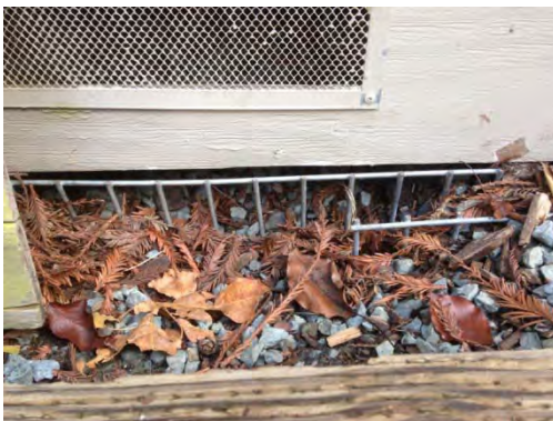
Dig Defense covering a gap under a portable building
