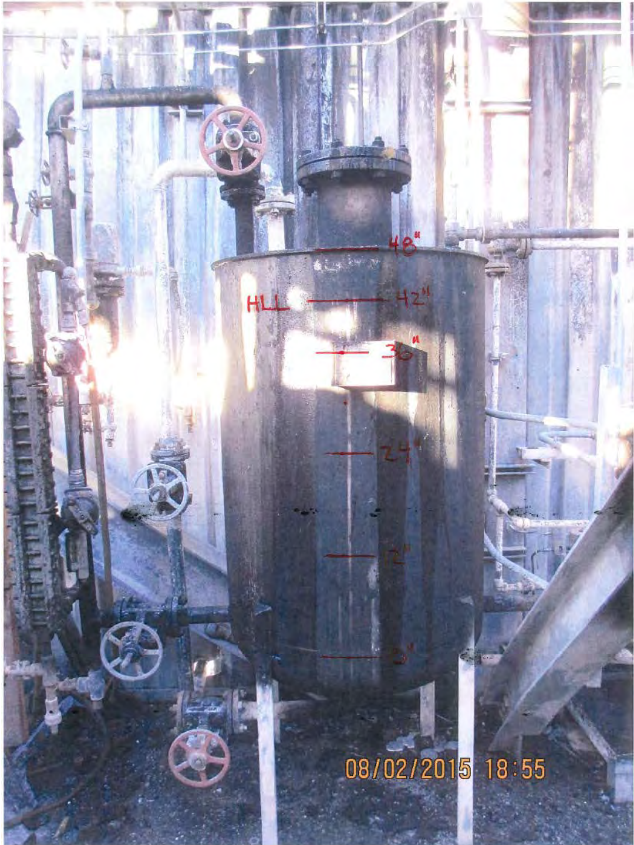
PICTURE OF DAY TANK WITH LEVELS MARKED
