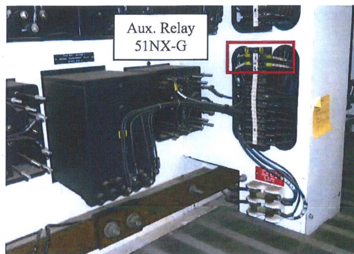
Figure 3 Wires on terminal strip at back of Panel 2
