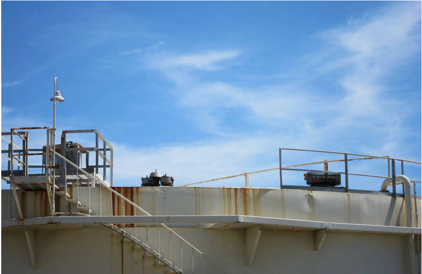
The Tank breather valves (PSV-294A & C) are visible to the right of the Gauger's Platform. The 20" Emergency Hatch is behind the railing at the right, near the 6" tank vent line.
