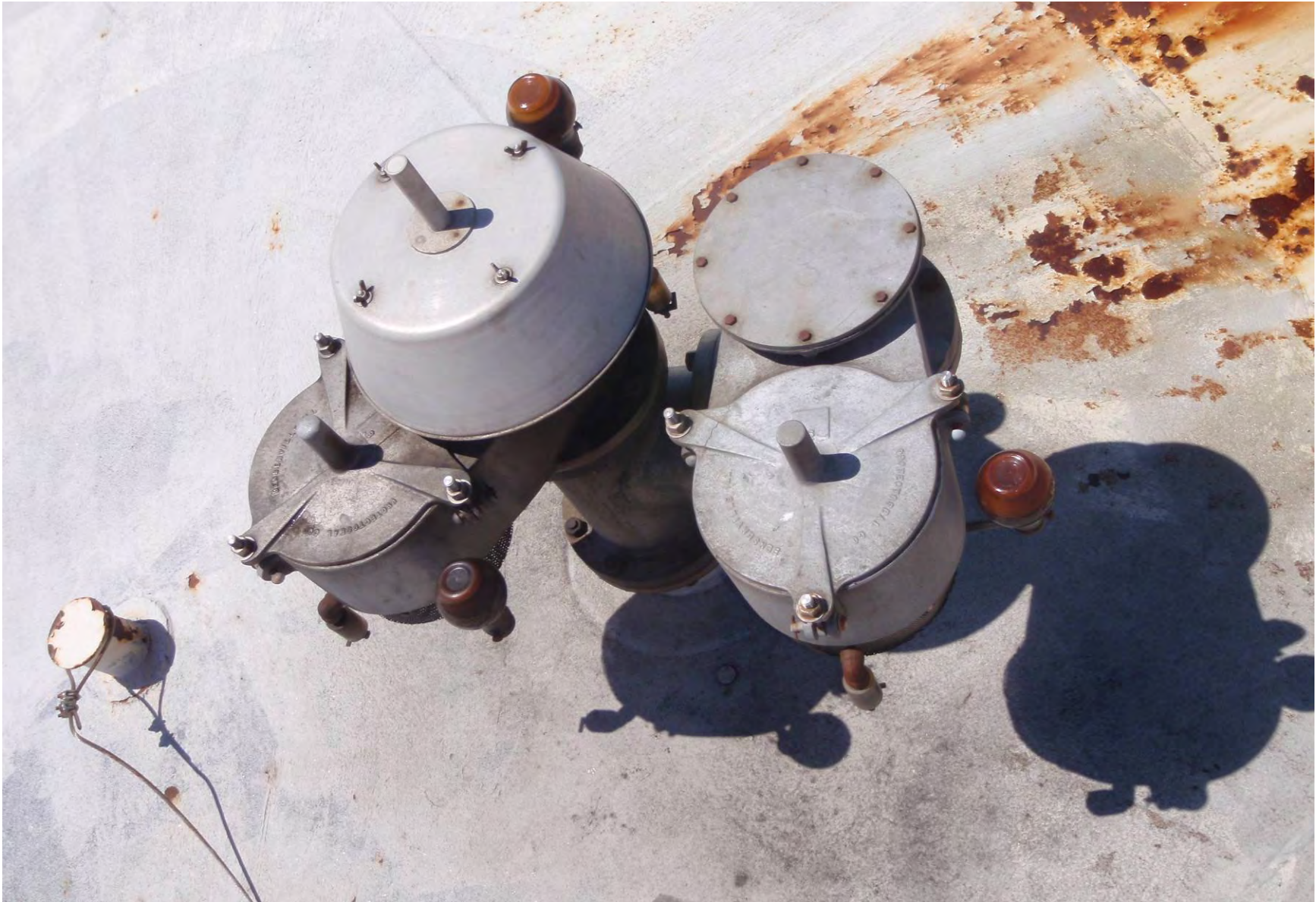
Close-up view of the Tank Breather valves (PSV-294A & C)
